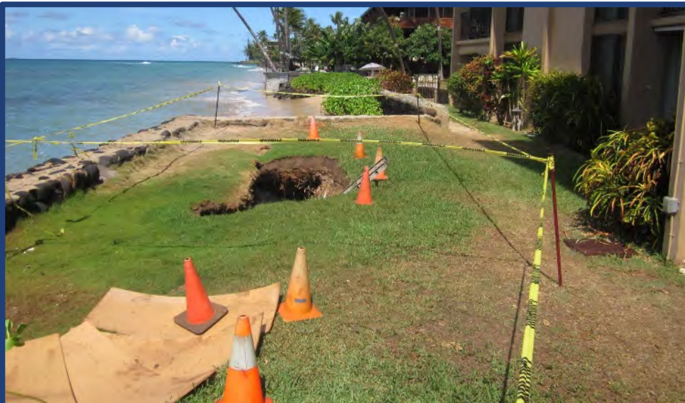
Figure 15. Example of a failing seawall and sinkhole caused by undermining from wave action and beach loss in West Maui (Tara Owens, Hawai'i Sea Grant).
